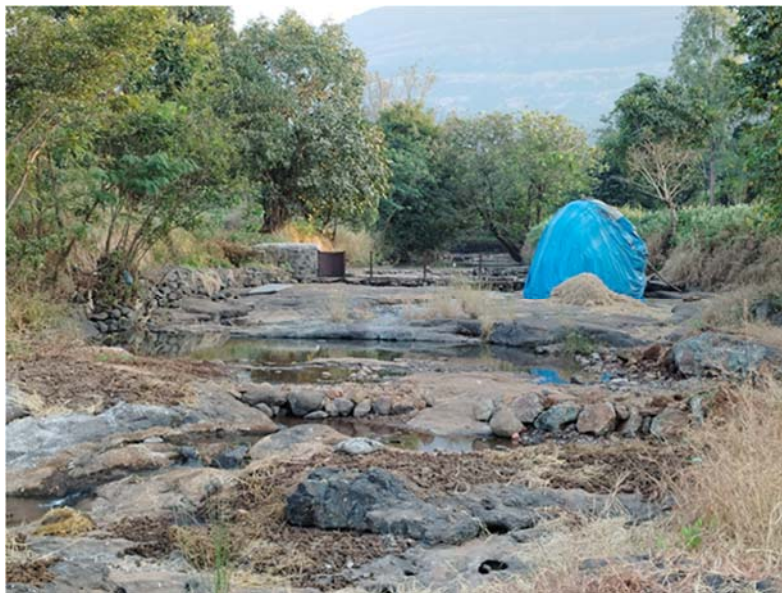
Picture 5.2: Washed away check dam on one of the streams in the Pavana catchment
